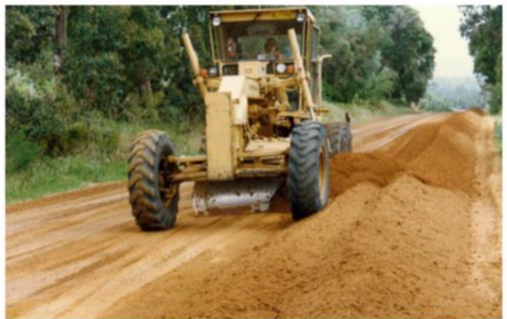
Grader mixing prior to more product and/or water alone to achieve optimum moisture content in the soil.
