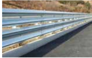
ROAD SAFETY GUARDRAIL
