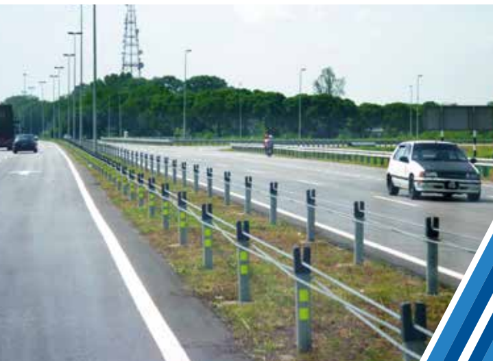
Installation at Permas Jaya, Johor Bahru, Johor
