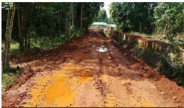
Soft and muddy condition – Difficult access
